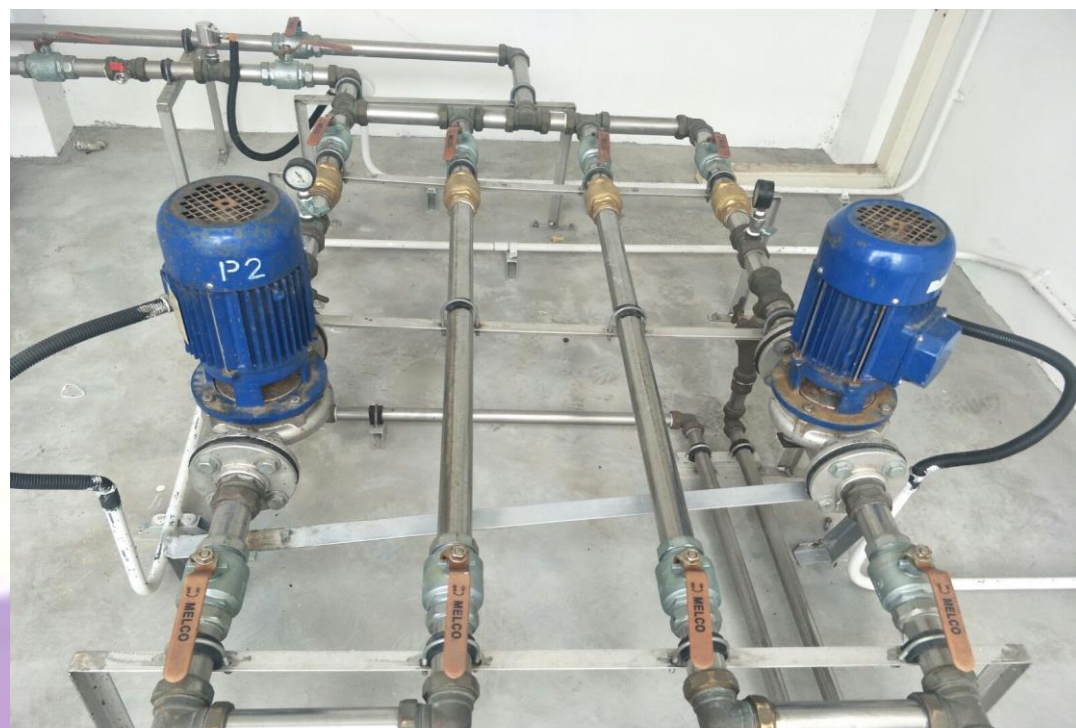
Replacement of booster pump sets and Refuse Chute Flushing System (RCFS) at Blk 101 to 120, 321 to 326, Blk 336 to 350, Blk 402 to 437(Marsiling)
